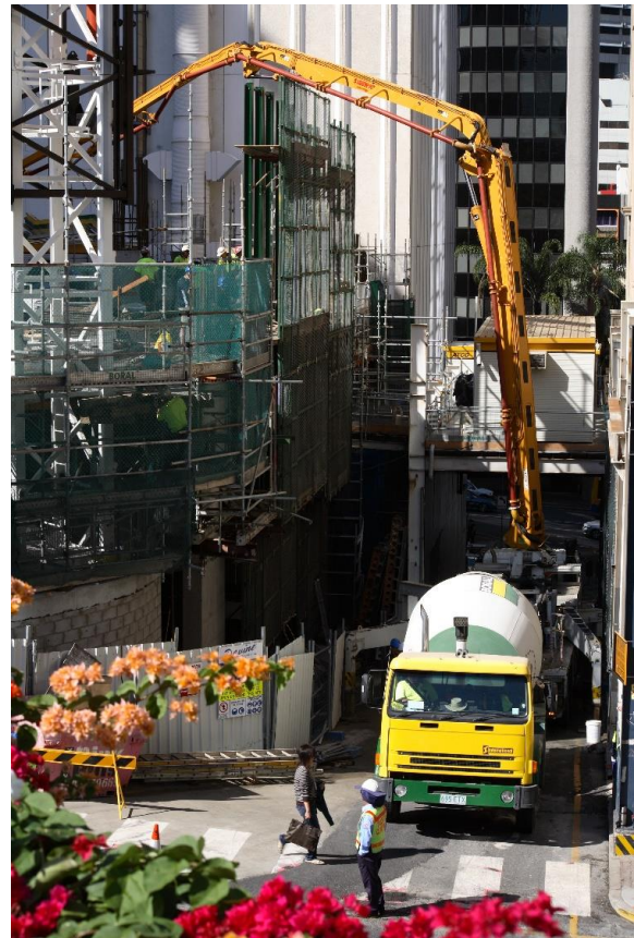
Figure 12.10 – Concrete Distribution by Pump (from a discharge point in street where permitted) is the Most Common Method
